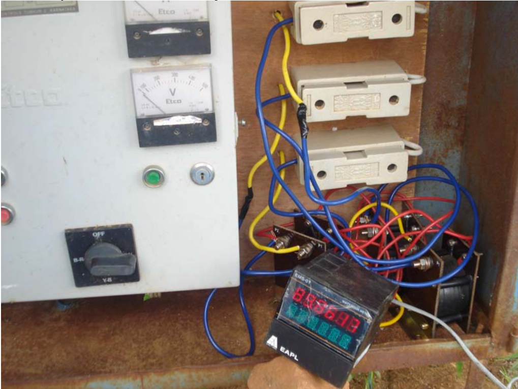
Electricity meter connected in a field
